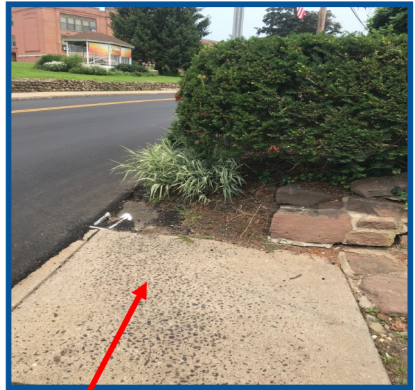
Figure 21: Abrupt end to Sidewalk
