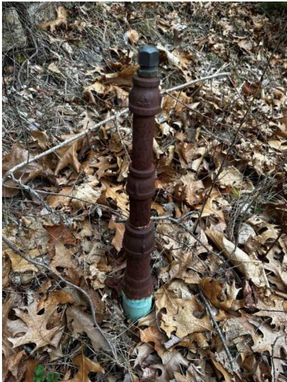
Valves located outside west side of gate house.
