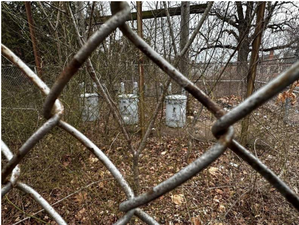
Three (3) pad mounted transformers
