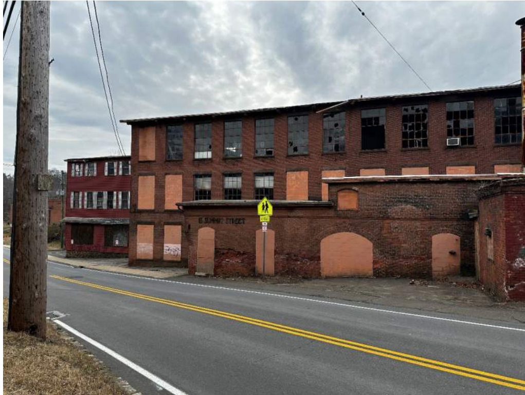
View of southern side of building along Summit Street. Former offices on left side of photograph. Former boiler house and a portion of the fire pump building on the right.
