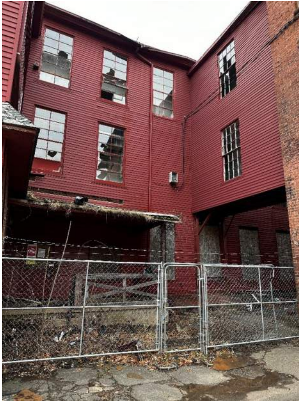
Two views of loading dock area between building at southwest side of building, looking north. Fence preventing access.
