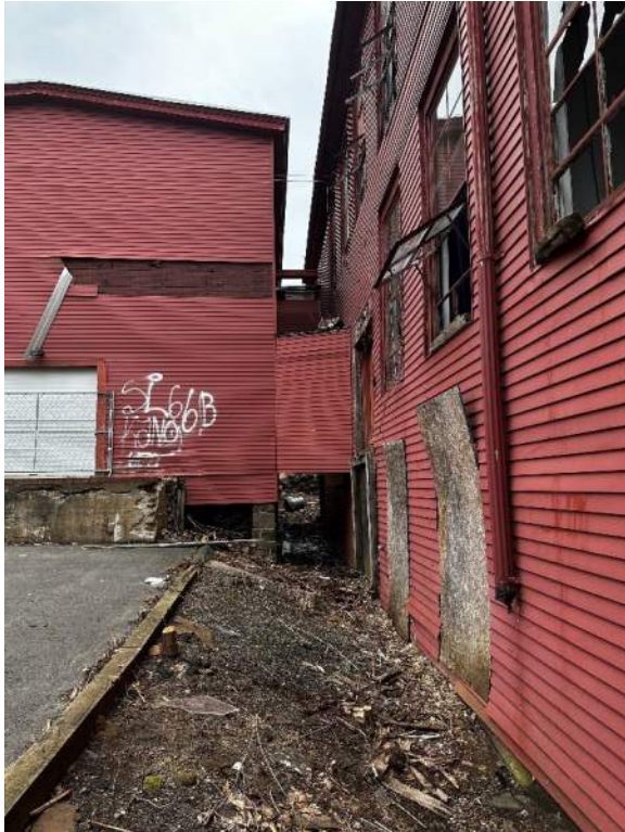
View of two interconnected buildings, looking east. Raised loading dock to the left of the photograph.
