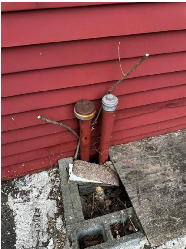
Fill and vent pipes at southwest corner of building
