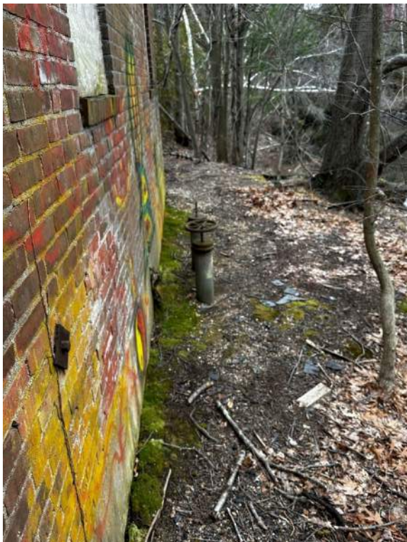
Valve located outside north side of gate house.
