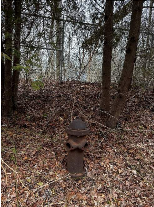
Out of service fire hydrant, north of westernmost portion of the building. Transformer pad in the background.
