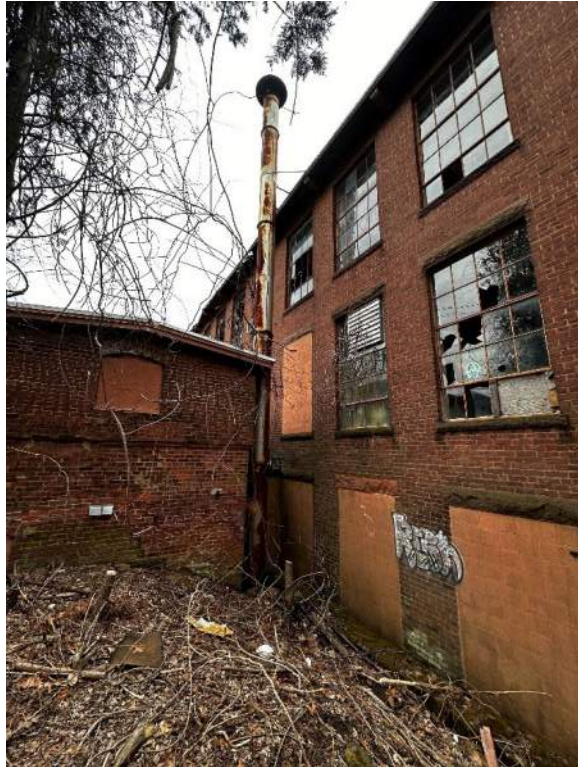
Two views of the area between two sections of the building, concrete lined and containing water and debris. The stone wall is part of the western boundary of Second Pond.
