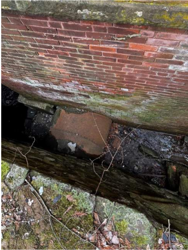
Two views of penstock and controls as they enter beneath the building at west end of Second Pond.
