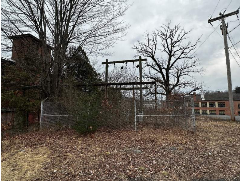
Pad mounted transformer area north of the building
