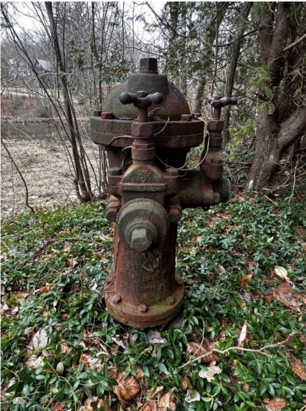
Fire hydrant on northern side of building
