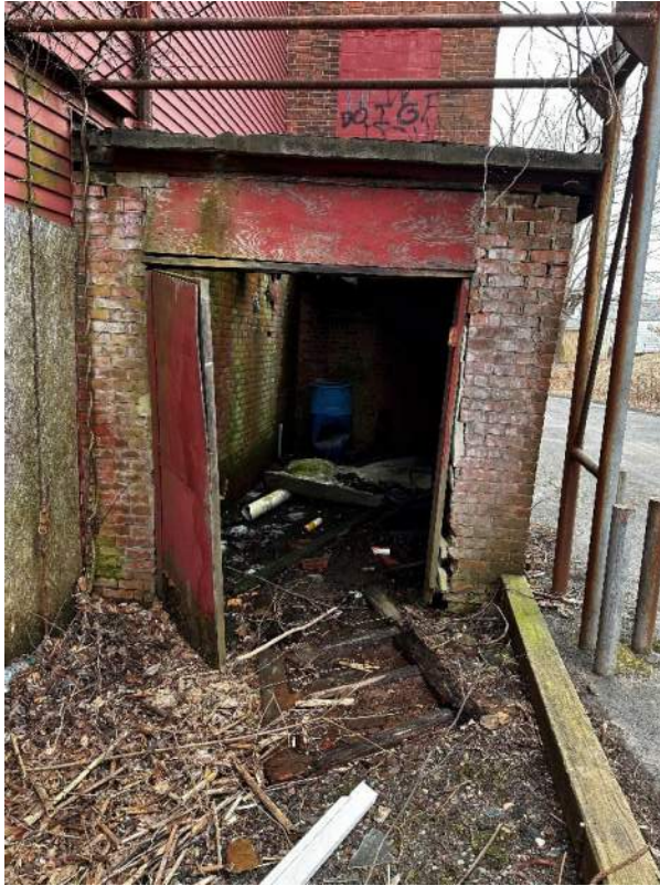
Two views at ground level of interior of multi-level elevator shaft on northern side of building.
