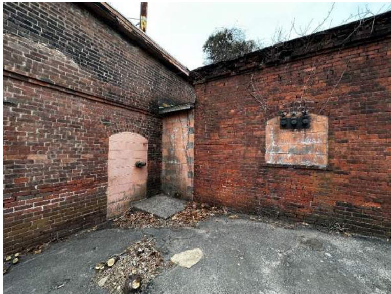
Western side of fire pump house.
