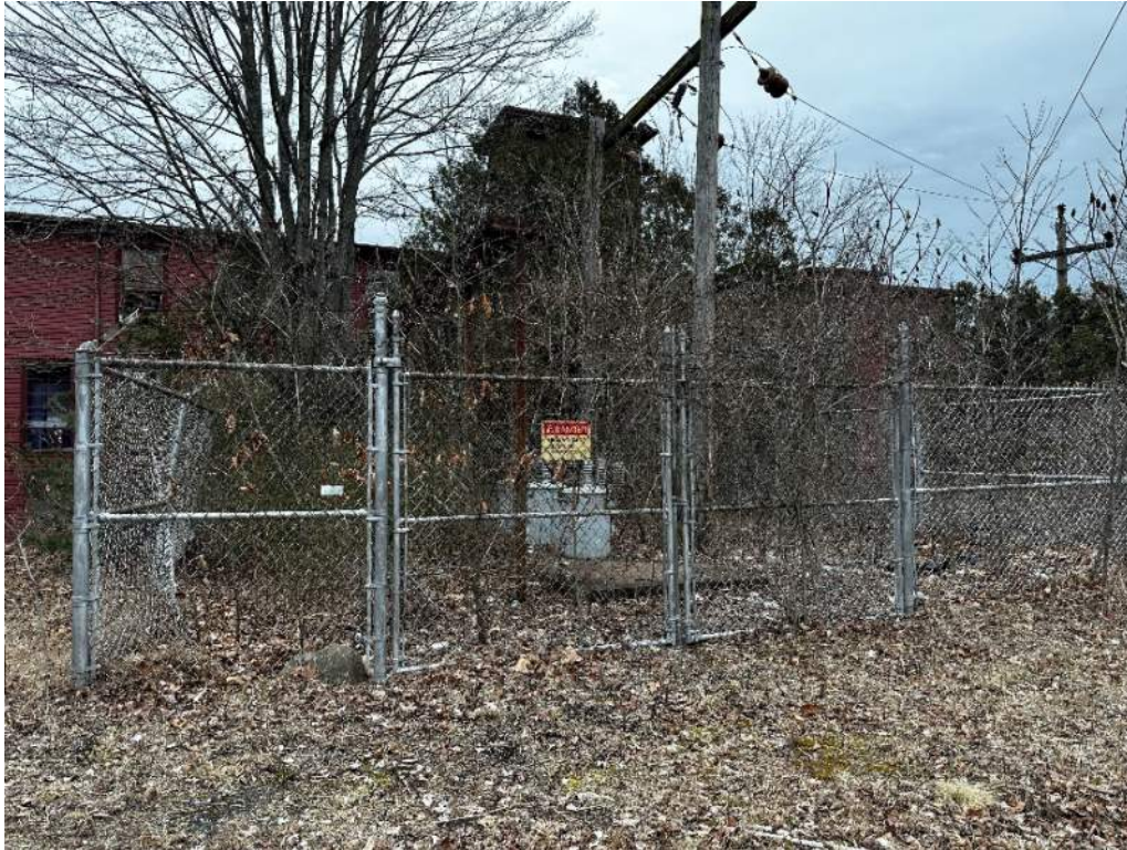
Pad mounted transformer area north of the building, looking south.
