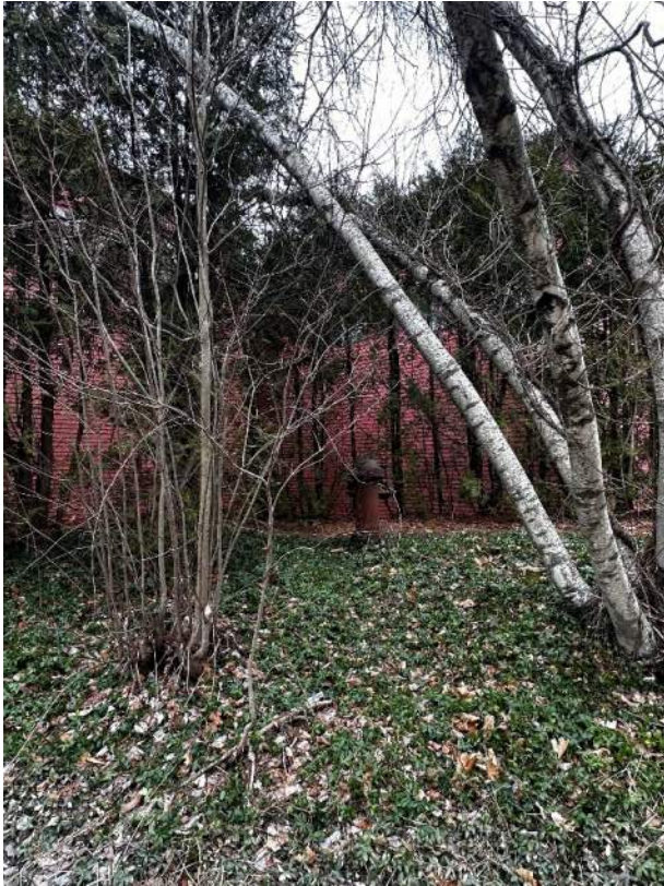
Fire hydrant on northern side of building.
