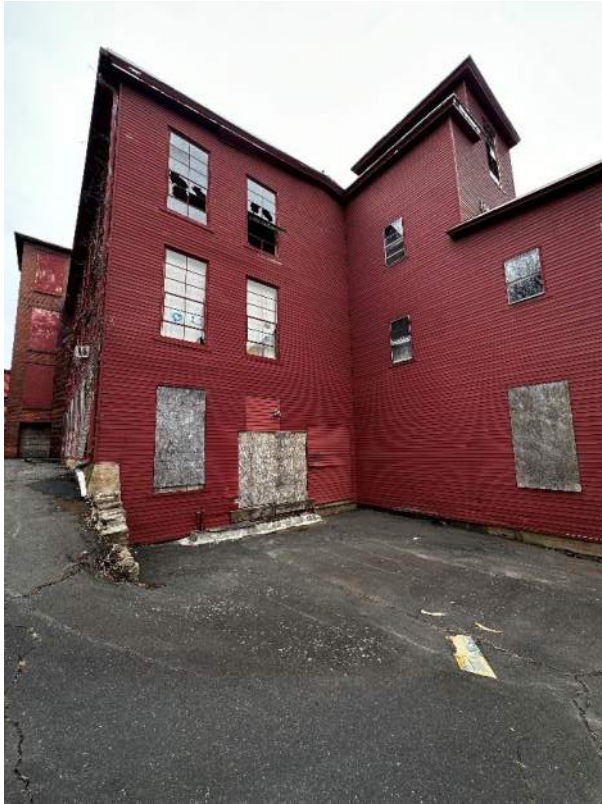
Area at southwest corner of building with fill and vent pipes visible, former offices, elevator and water wheel. Vent and fill observed beneath lower left window.
