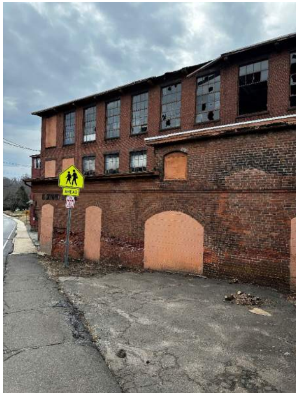
Former boiler house and manufacturing building in rear, looking northeast. Summit Street on left side of photograph.
