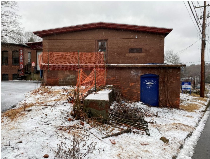
24: View of northeastern portion of building, looking from corner of Summit Street and Starr Place. Orange construction fence surrounding portion of a 1 st -story roof that has fallen.
