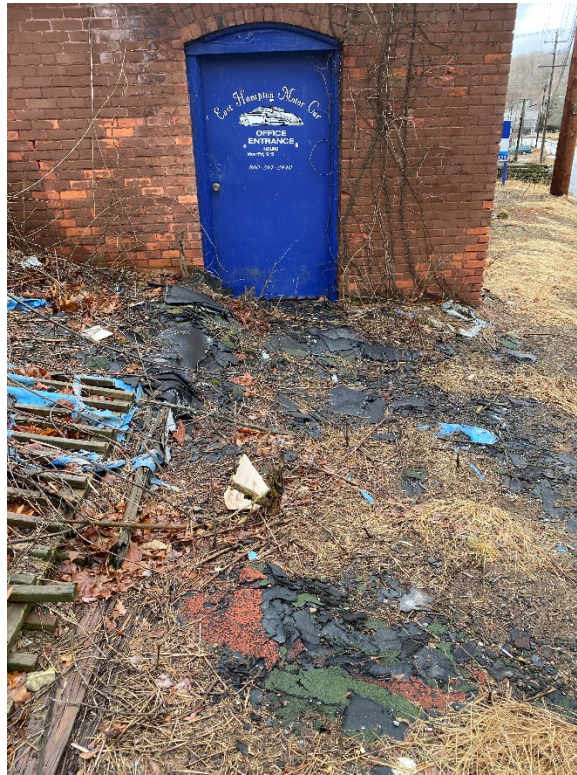
25: View of northeastern portion of building, roof shingles on the ground
