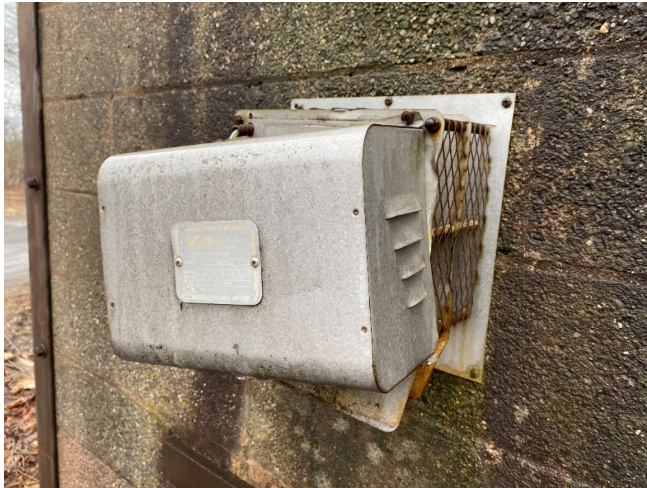
16: Sidewall power vent, at southeast corner of building
