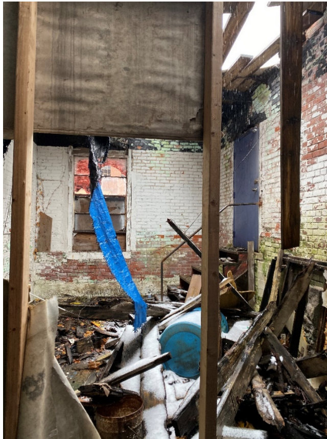
45: View of 1 st -story room at northernmost portion of building, with a fallen roof.
