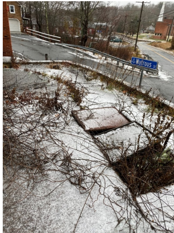
4: View of location of an apparent underground storage tank, corner of Watrous and Summit Streets.
