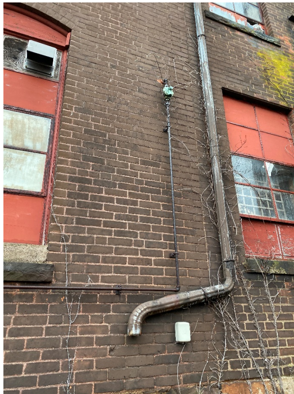
10: Gas regulator and piping on western side of building (near former water tower)
