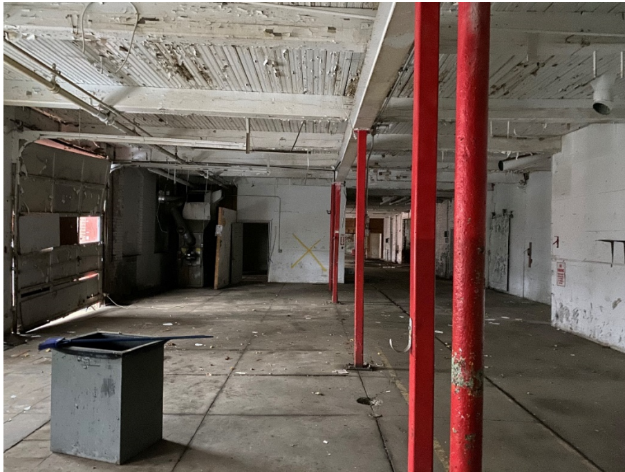
35: View of 1 st -story room, concrete floors, wooden ceilings, floor drain trench on inside of overhead door.
