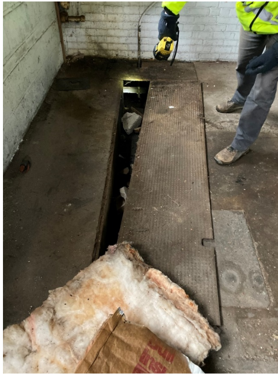
47: View of 1 st -story entry, possible vehicle repair area, with floor drains.
