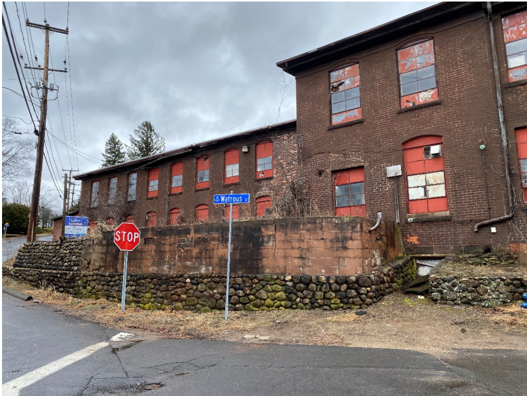
3: View of location of an apparent underground storage tank, corner of Watrous and Summit Streets.
