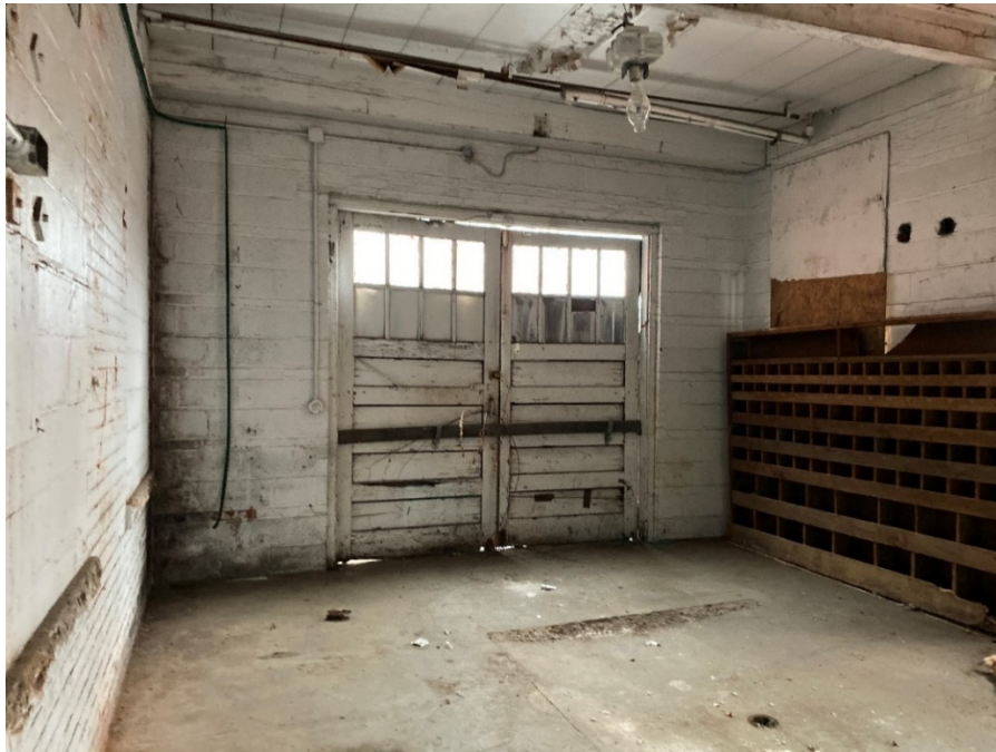
46: View of 1 st -story entry, possible vehicle repair area, with floor drains.
