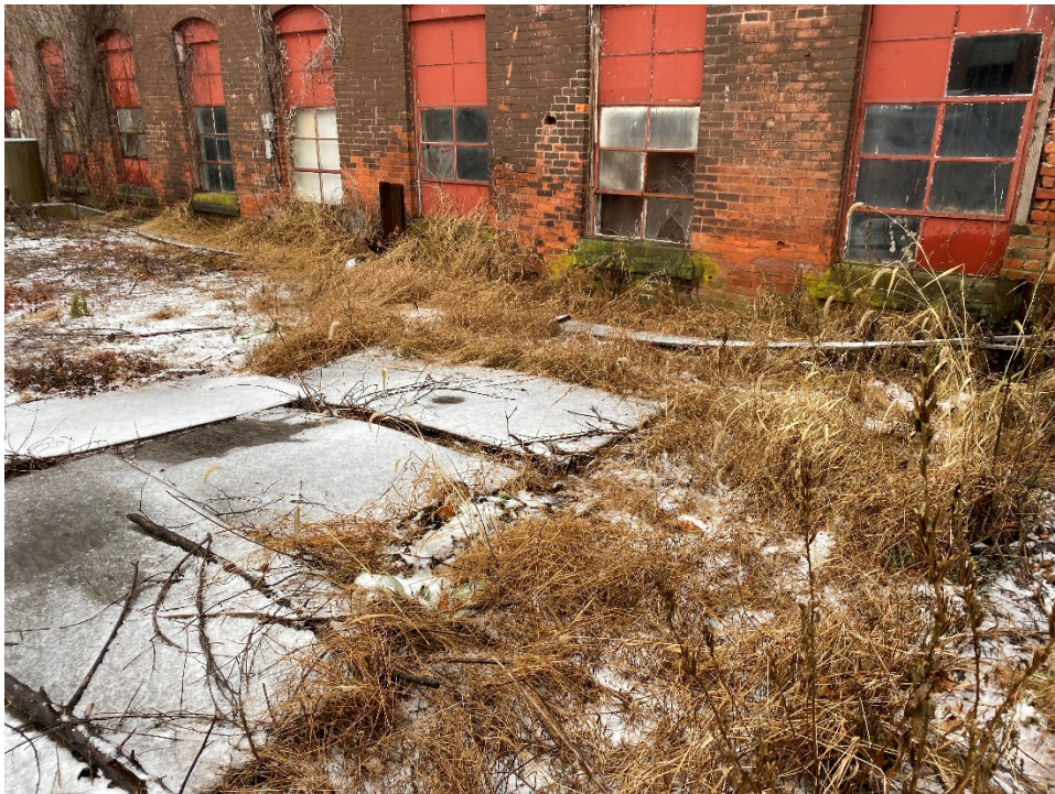
8: View of location of former Water Tower area on north side of building.
