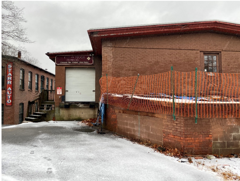
23: View of loading dock at northeastern corner of building, looking from Starr Place. Orange construction fence surrounding portion of a 1 st -story roof that has fallen.
