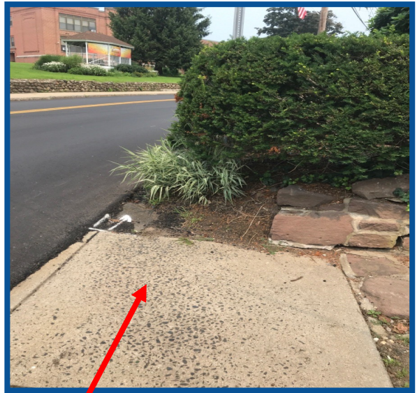
Figure 21: Abrupt end to Sidewalk
