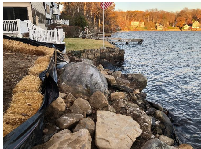
Bank stabilization at southern property boundary. Wetland boundary comprised of OHW line to Pocotopaug Lake.
