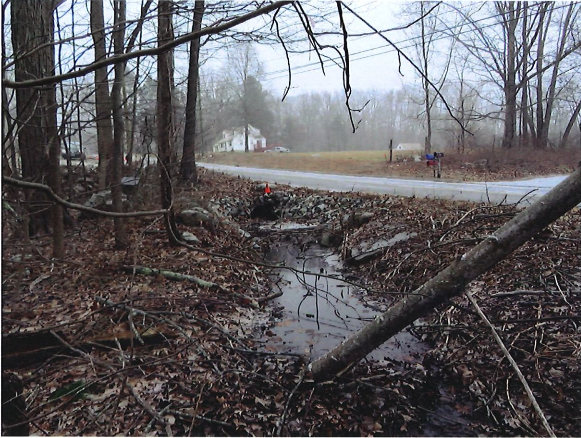
Photo 3: Stormwater Outfall & Associated Basin adjacent to Cone Road
