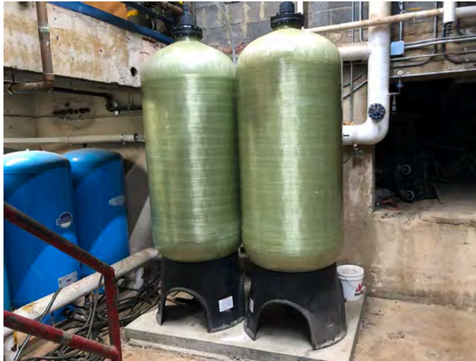
Photo 5: Treatment Facility at the Memorial School
