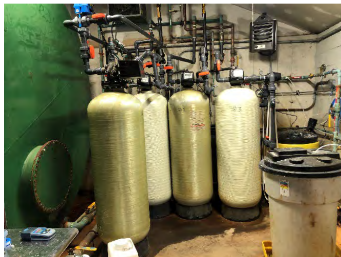
Photo 4: Treatment Facility for the Royal Oaks System
