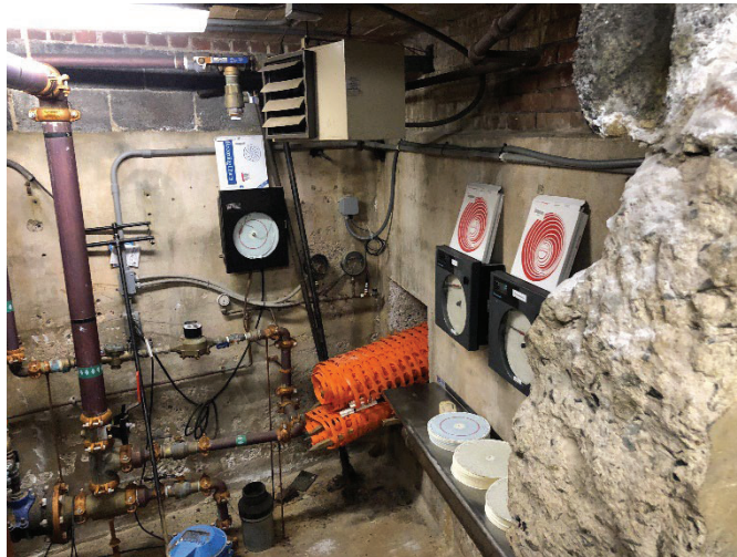
Photo 3 – Treatment Facility for the Village Center System
