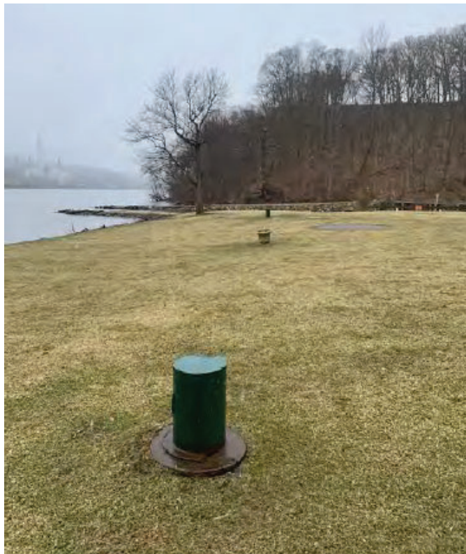
Photo 3-5 – Cobalt Landing Wellfield Capped Wells
