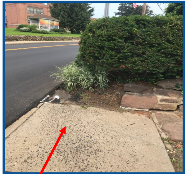
Figure 21: Abrupt end to Sidewalk
