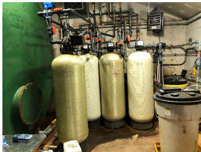
Photo 4: Treatment Facility for the Royal Oaks System
