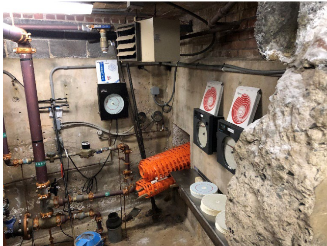
Photo 3 – Treatment Facility for the Village Center System
