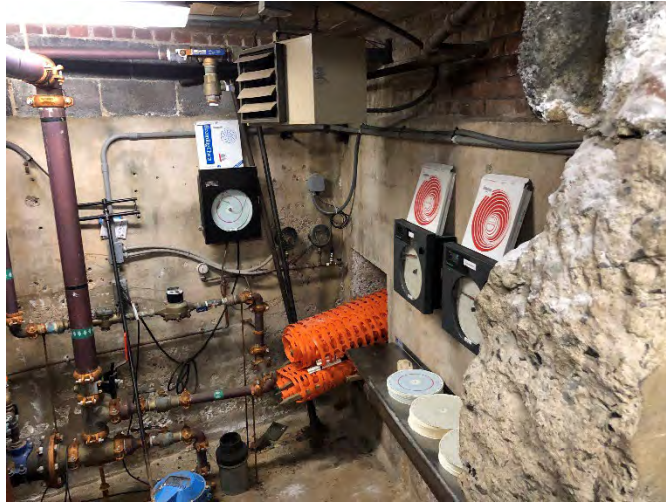
Photo 3: Treatment Facility for the Village Center System
