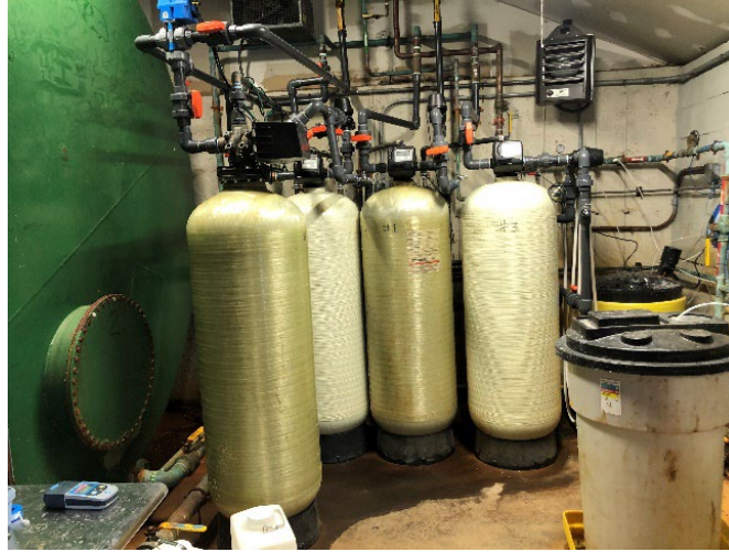
Photo 4 – Treatment Facility for the Royal Oaks System
