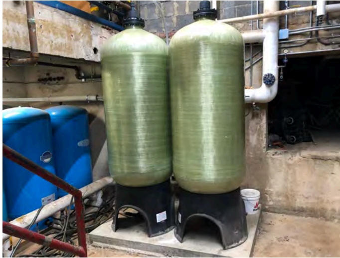
Photo 5: Treatment Facility at the Memorial School
